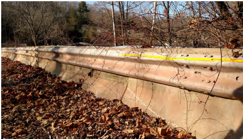
Figure 2 Jersey barrier on Headquarters Road Bridge, showing impact scrapes, possibly resulting from the 24 October 2003 crash
